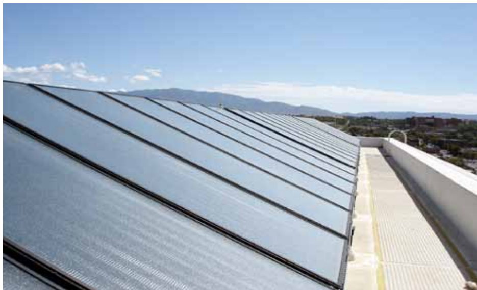
Solar Panels Produce 60% of Hotel's Domestic Hot Water Needs
